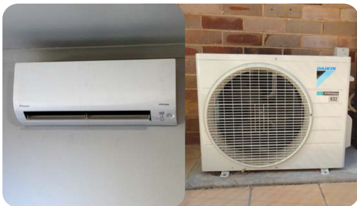
A reverse-cycle split-system heat pump provides efficient heating and cooling.
