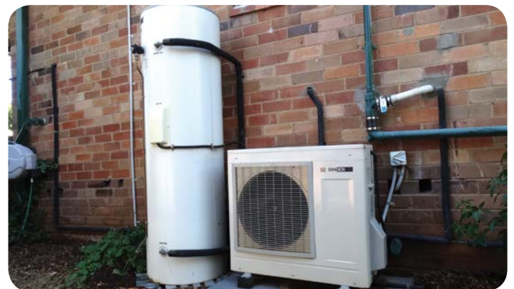
A heat pump hot water system will deliver hot water cleanly and efficiently.
